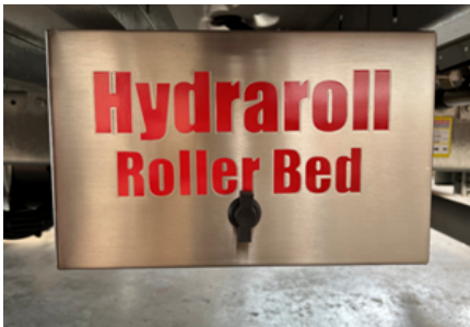
Roller control panel
