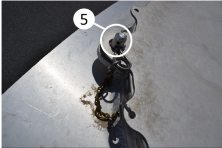
Manhole sealing cover
