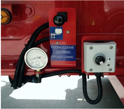
Hydraulic control panel
