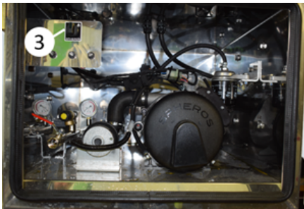
Switch in cabinet
