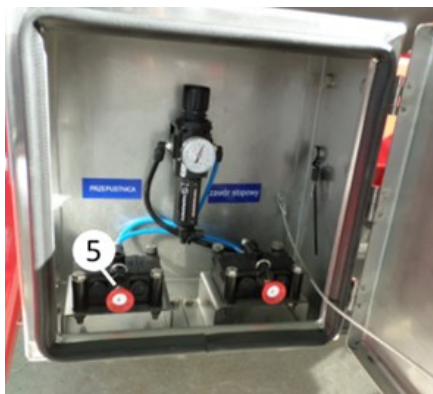
Pneumatic control box
