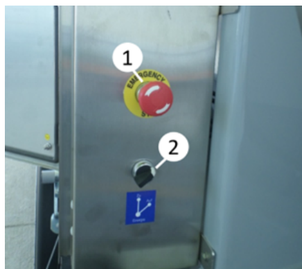
Panel de control
