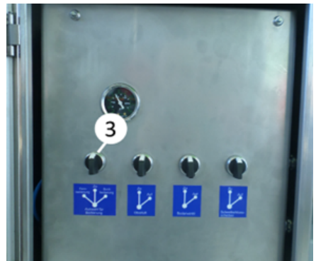
Panel de control
