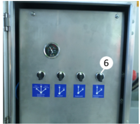
Panel de control
