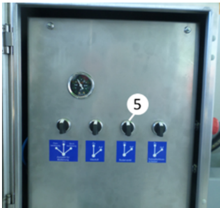
Panel de control
