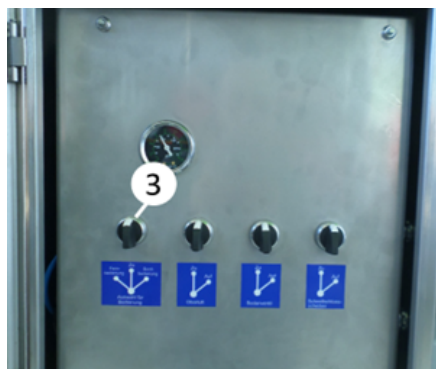
Panel de control
