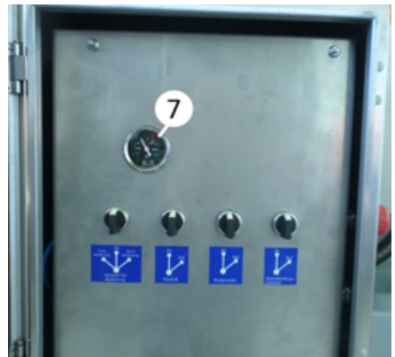
Panel de control
