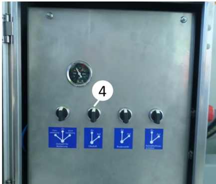
Panel de control
