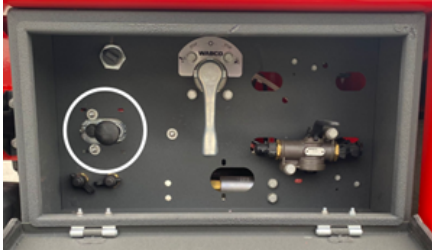
Axle lift button on control cabinet
